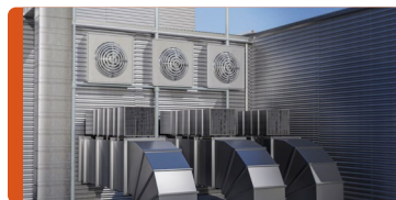
Central air conditioner
